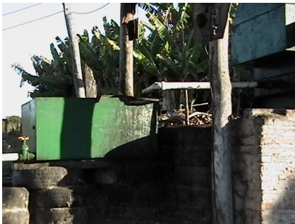
Figure 2e. Dilution tank
